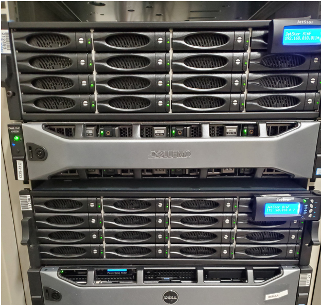
Two AC&NC JetStor SAS 816F Arrays at the Beach TV data center
