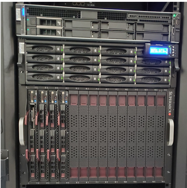
The third AC&NC JetStor SAS 816F Array at the Beach TV data center
