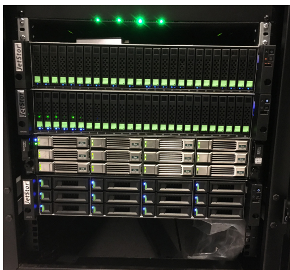
The JetStor 826iXD All Flash Array , JetStor 826JXD All Flash JBOD , and JetStor 812iXD Array at StratusLIVE’s remote data center
