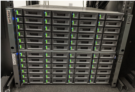
The JetStor 824iXD Array and JetStor 824JXD JBOD at Miller Electric’s data center
